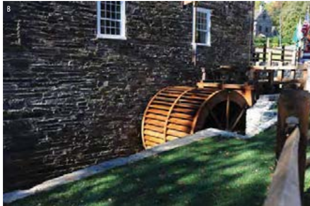
Peirce Mill, construction of new flume Peirce Mill, installation of new wheel Arts & Industries Building restoration
