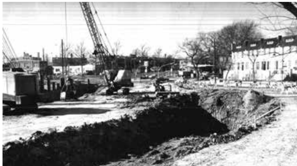
Construction for the Southeast Freeway disrupts the setting of Barney Circle District Department of Transportation
