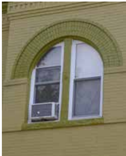
Windows do not fit arched masonry opening
