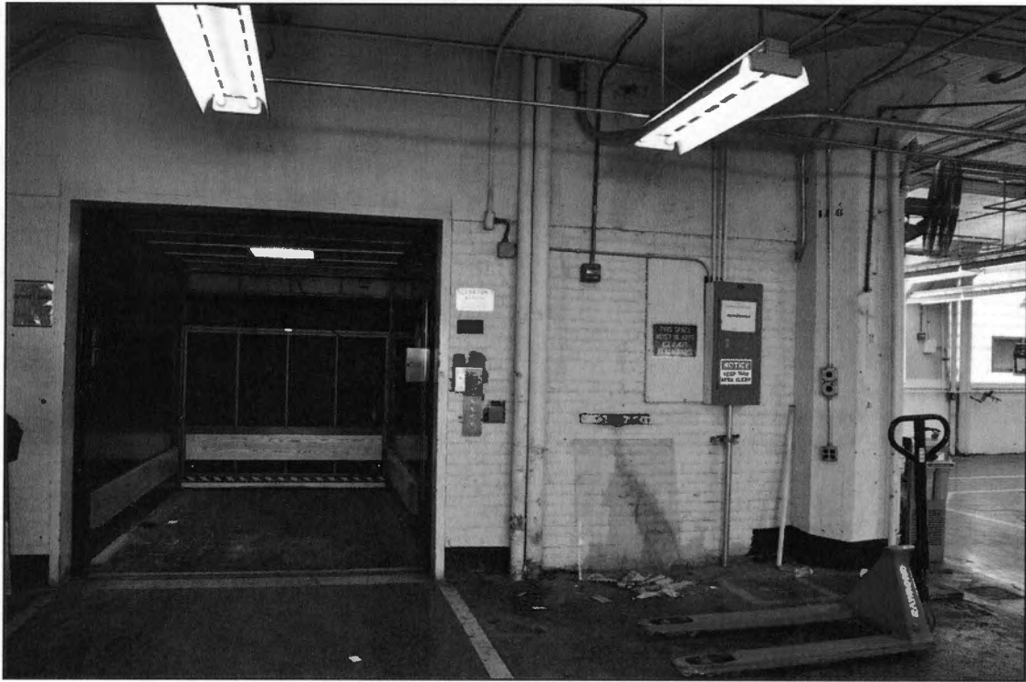
PHOTO 16: First Floor, View of Elevator No. 1
