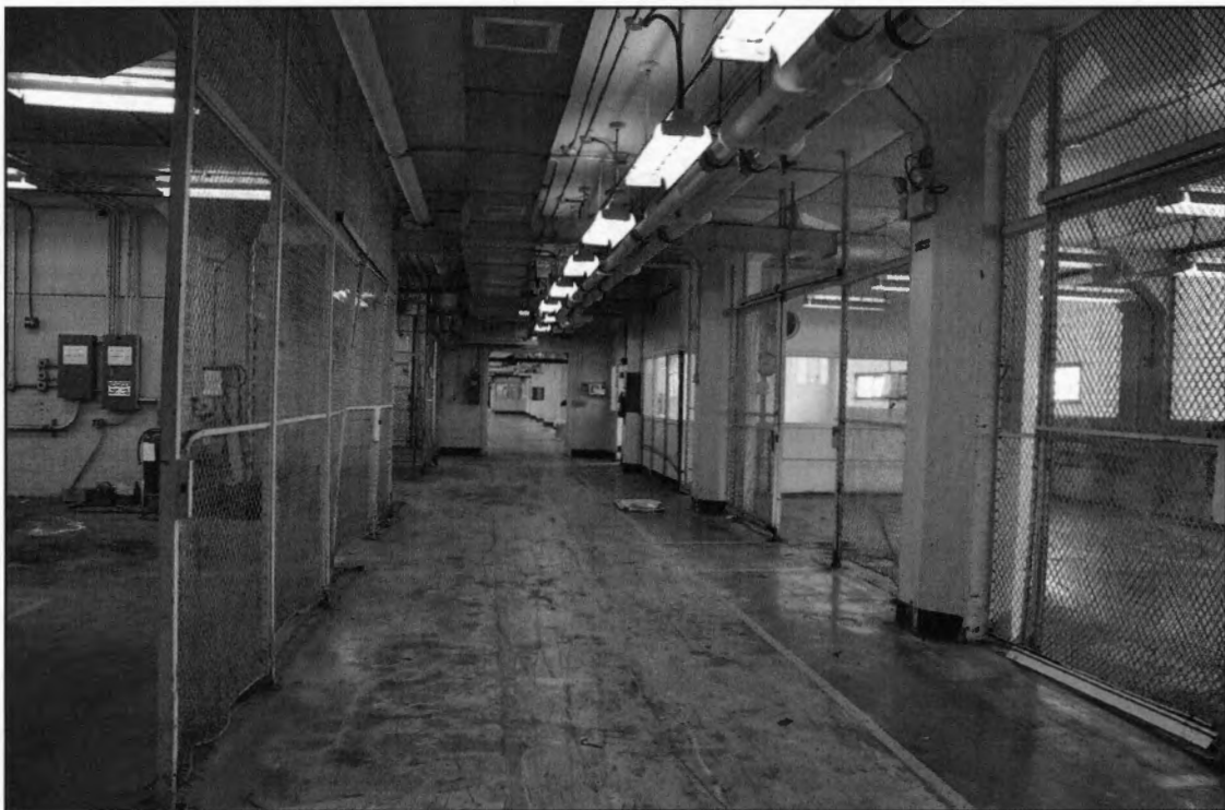
PHOTO 21: Second Floor, East Portion Of Building, Corridor Looking East Toward Storage Areas
