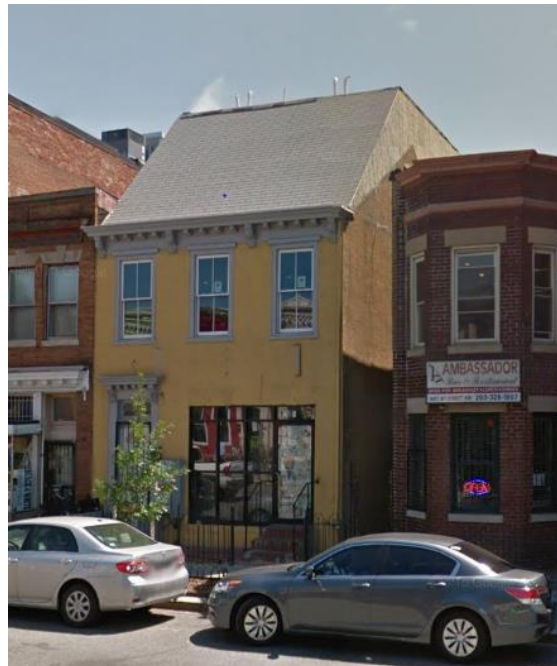
After roof alterations. Note the ghost mark on the side wall showing the original building outline.
