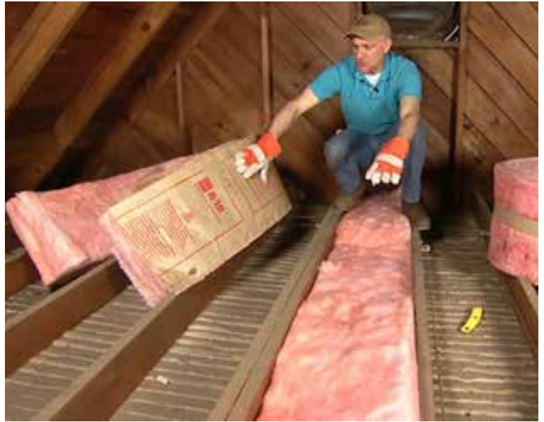
BATT INSULATION BETWEEN THE CEILING JOISTS
