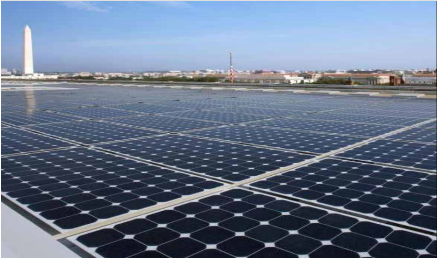
SOLAR PHOTOVOLTAIC SYSTEM ON THE JAMES V. FORRESTAL BUILDING, HEADQUARTER OF THE US DEPARTMENT OF ENERGY.
