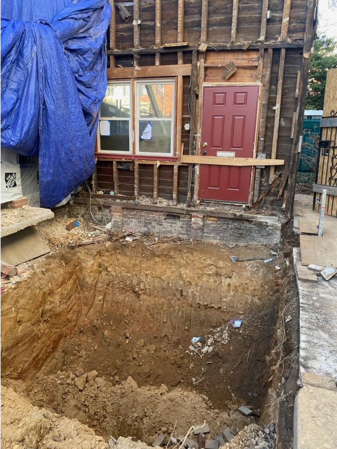
639 A Street SE showing back of front façade (photo courtesy of property owner)
