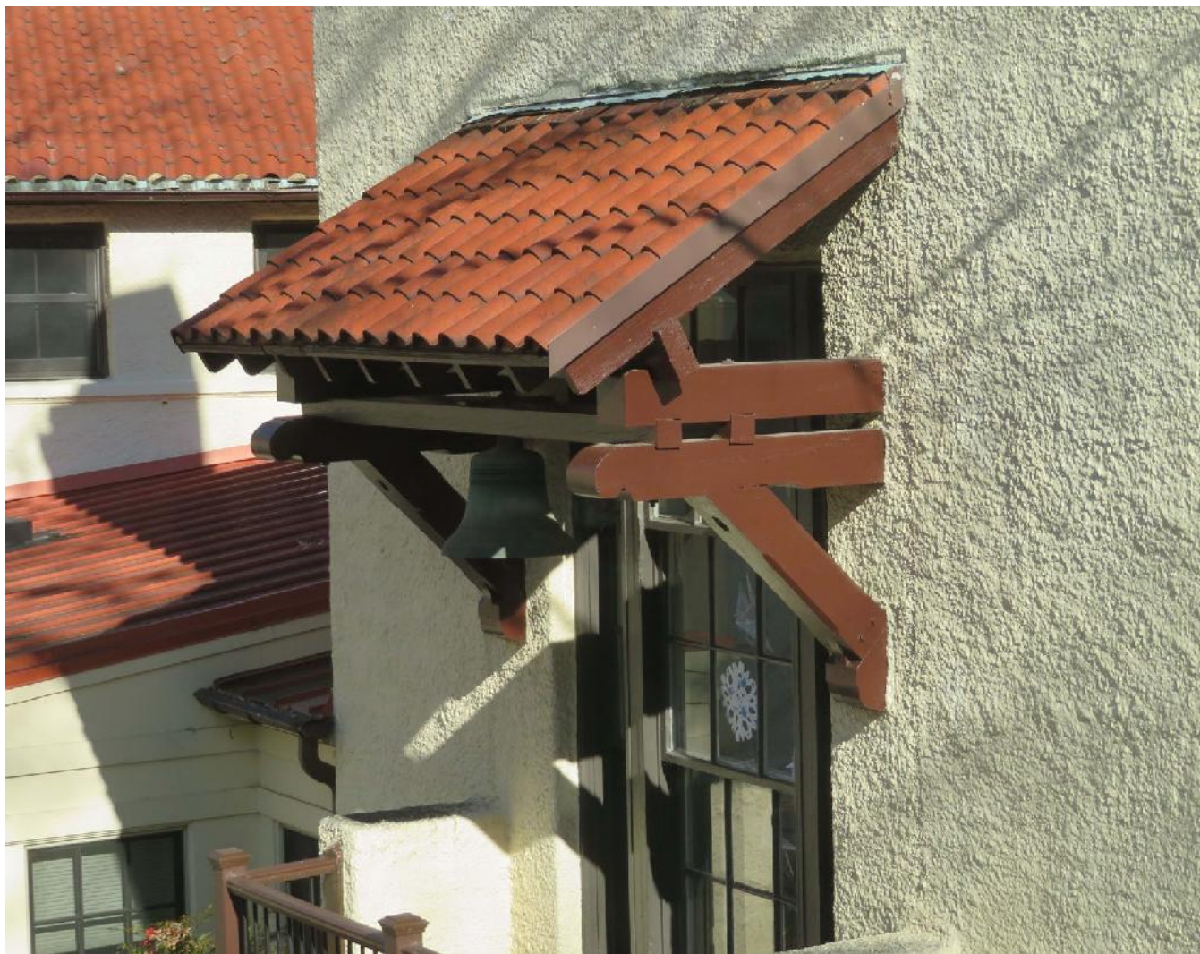
Photo 13: Rosemount Center, Main Block Rear Façade, Balcony Roof Framing detail (J. DeFerrari).
