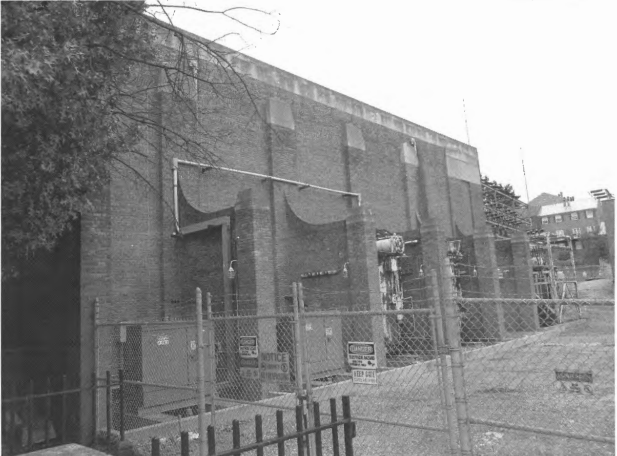
Pepco Substation No. 25
