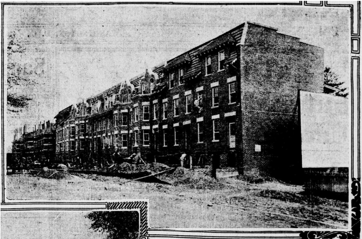
South side of the 700 block of Rock Creek Church Road. View east from Georgia Avenue showing houses in the course of construction. From The Evening Star , March 26, 1910, pt. 2, p. 2.
