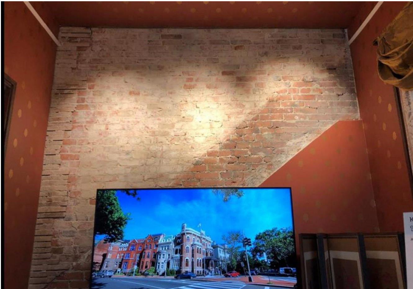
Photo 12: First floor interior, former servants' quarters and butler's pantry, now an orientation room, looking south. Ghost of former servants' stair exposed during restoration.
