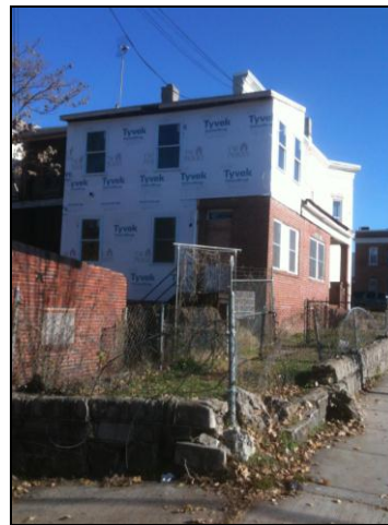
Current view of the south/west sides with partly completed addition. Source: OP.
