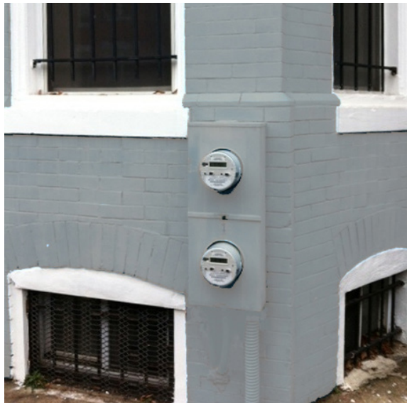
Painted electrical meters
