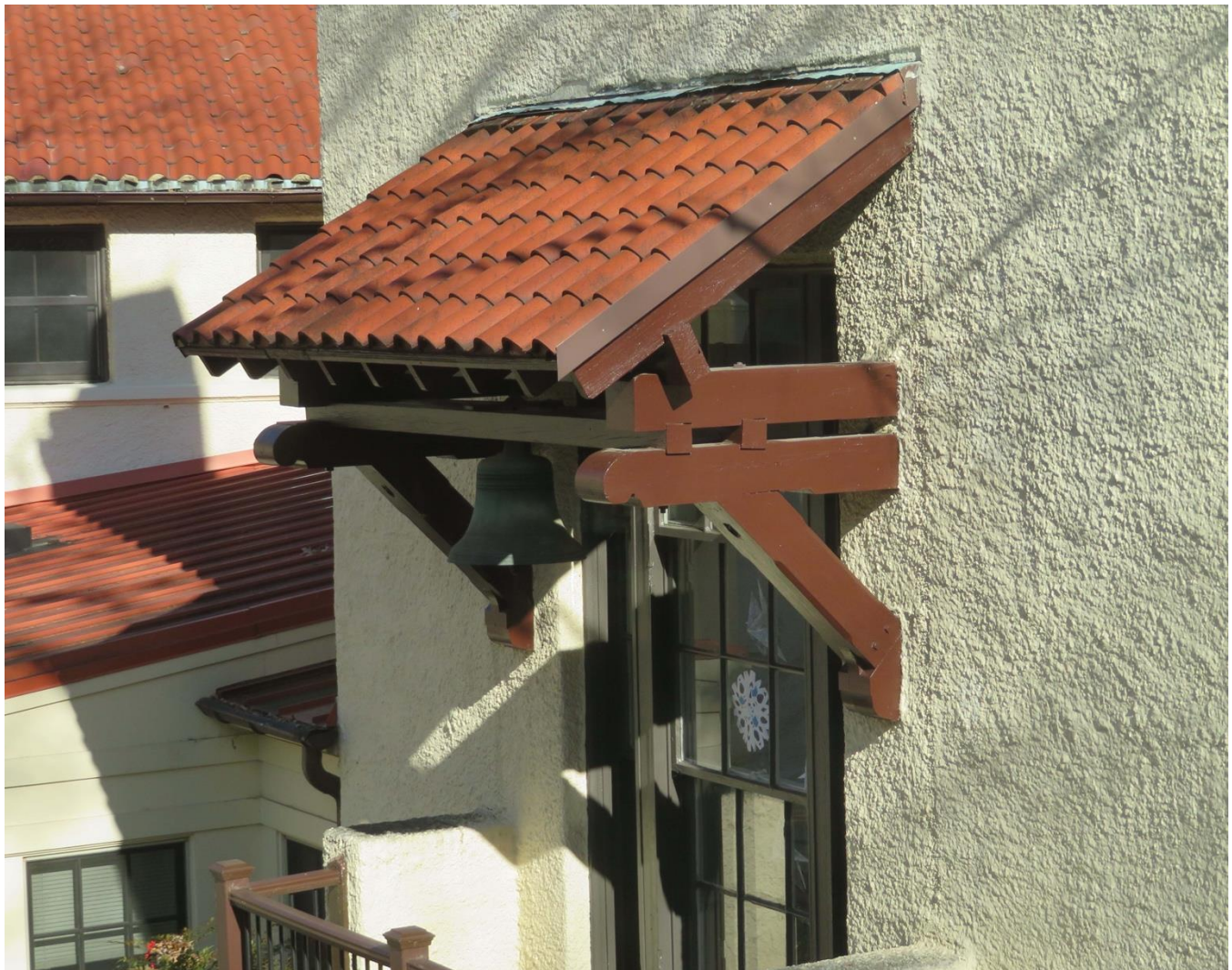
Photo 13: House of Mercy, Main Block Rear Façade, Balcony Roof Framing detail (J. DeFerrari).
