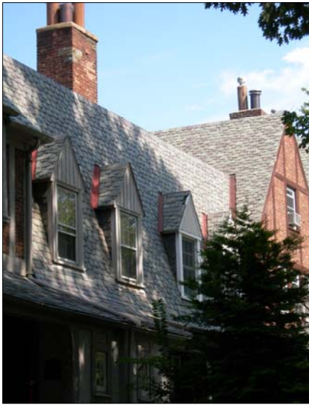
The slate roofs of houses in Foxhall Village were laid in subtle patterns that should be replicated in any replacements.
