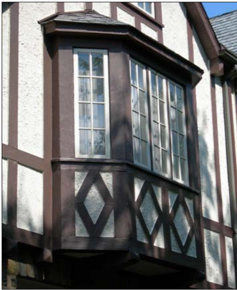
The first option for historic windows should be repair rather than replacement.
