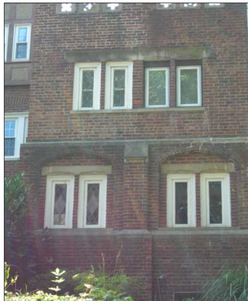
The replacement of historic windows with new windows that fail to match the details, configuration, and finish of the originals results in the loss of a significant architectural feature.
