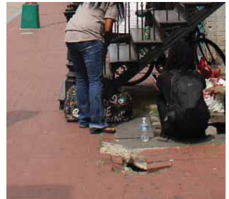
Sidewalk on H Street in disrepair
