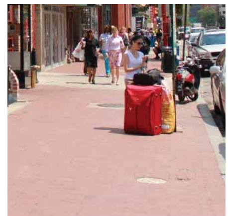
Missing decorative pavers on H Street
