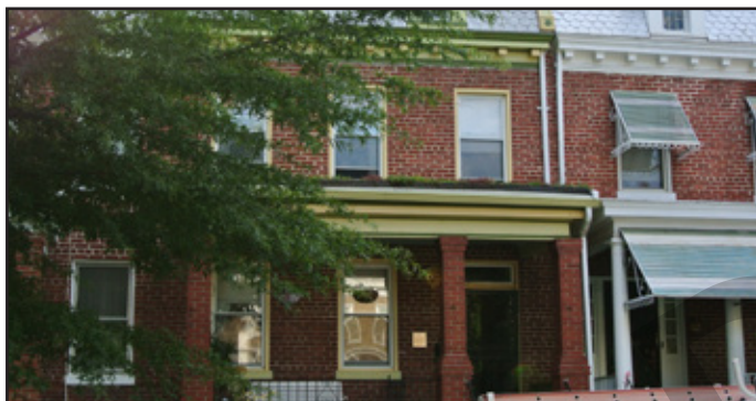
This green roof is installed on the porch roof, with high visibility from the street. The underlying waterproof membrane is visible below the plant materials.
