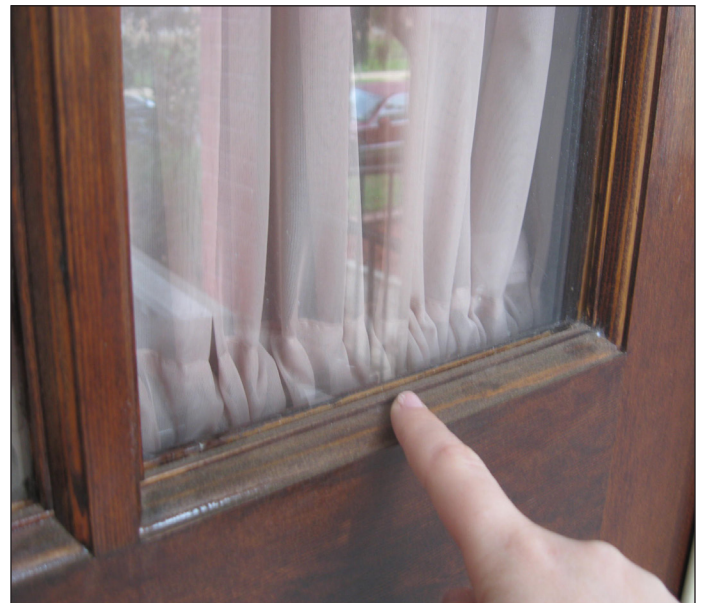
This door has wood molding around each pane that can be removed for the insertion of replacement glass.
