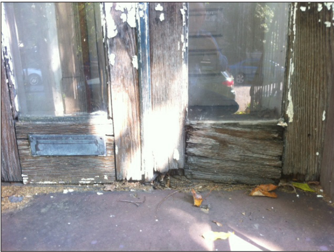
The bottom rail and side stiles of these doors are severely deteriorated, requiring reconstruction with new wood elements or wholesale replacement.
