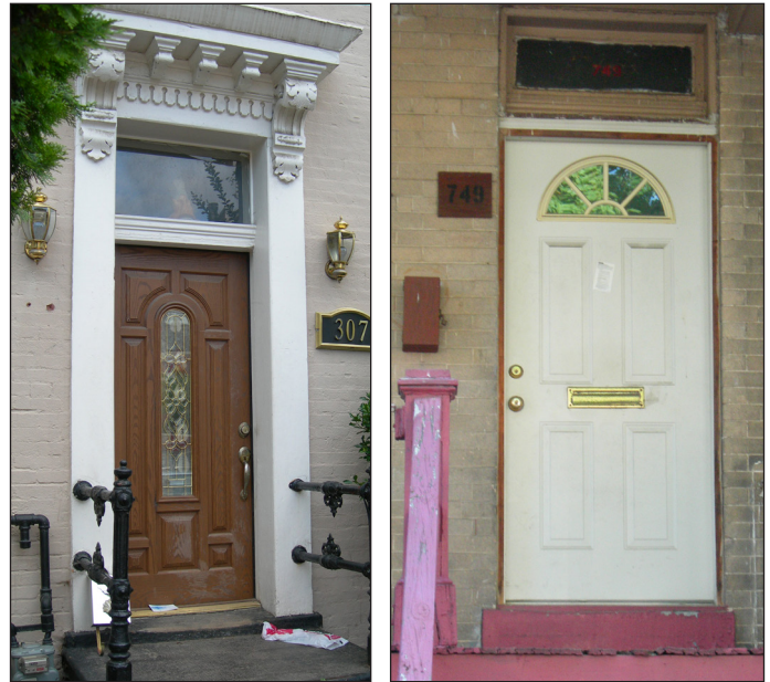
The unusual panel configuration and faux-leaded glazing of the door on the left, and the fanlight glazing in the door on the right have no historical precedent and are not compatible replacements for historic properties.
