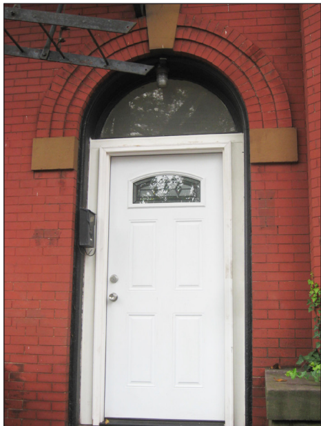
This replacement door is not compatible with the character of the building and not properly sized to fit the opening.
