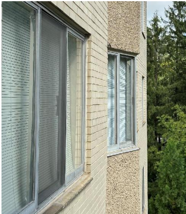
Figure 4: An example of the canted bays with aggregate concrete panel details. Photo by EHT Traceries.
