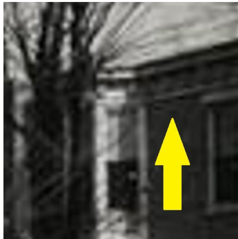
A cornice existed on the former rear addition. It was moderately decorated with modillions. (Image from DC Public Library).
