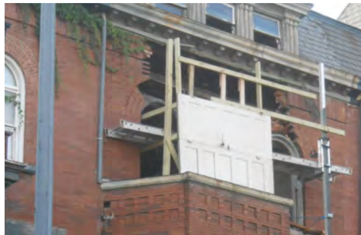
2212 1ST STREET NW - BEFORE
