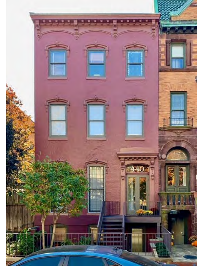
NEW FLEUR DE LYS CAST FROM THE ORIGINAL FOR FACADE RESTORATION - 440 M STREET NW
