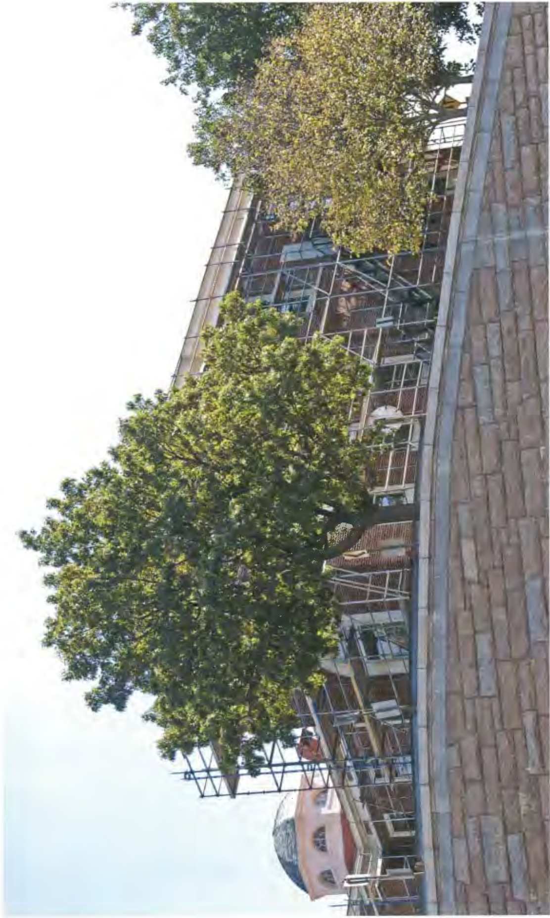
Image B4: Central Building, west façade of west hyphen with painter's scaffolding in place, looking NE from E Street Freeway entrance ramp.
