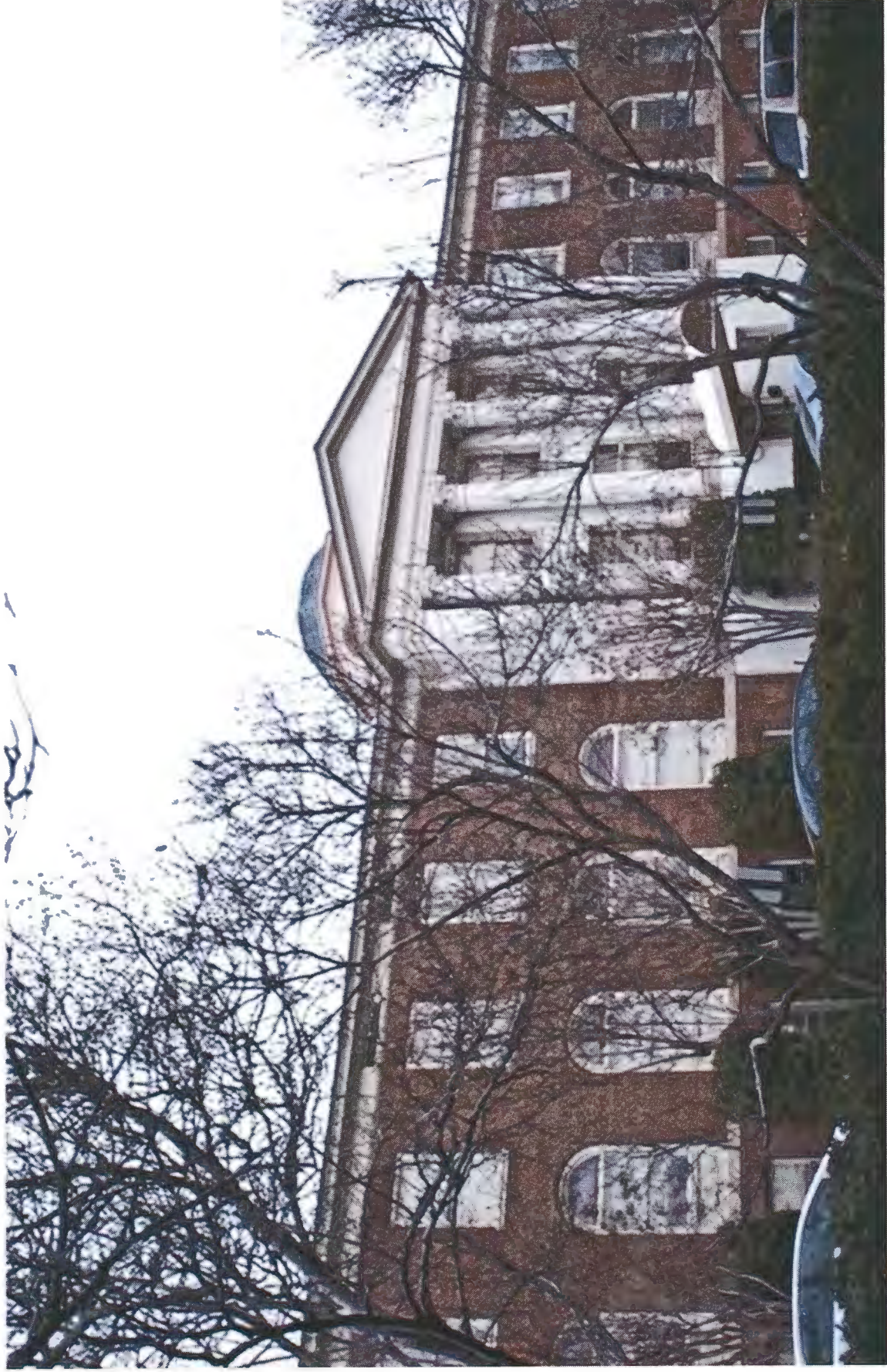
Image B5: Central Building, west section of south façade, looking northwest from quadrangle.
