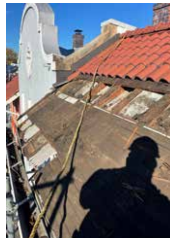
MOUNT PLEASANT ROWHOUSE DETERIORATED ROOFING AND EAVES
