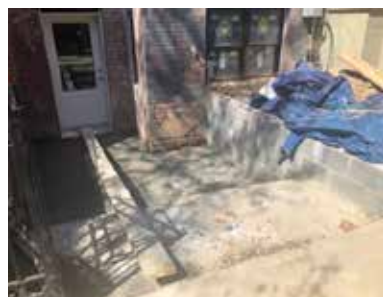
UNPERMITTED SITE WORK IN PROGRESS
