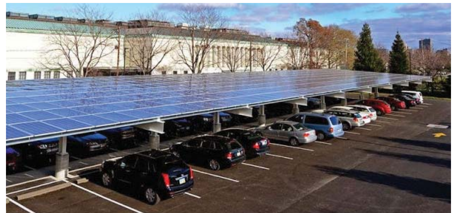
SOLAR ENERGY ©PS Pascal Steel
