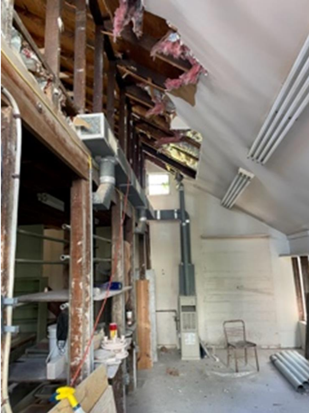
Interior of outbuilding at 515 Cedar showing older wall framing and newer roof framing. The older framing elements are of different sizes, possibly indicating that they were reclaimed and reused.
