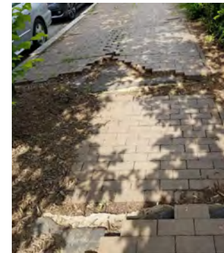
Paths and Benches in Disrepair
