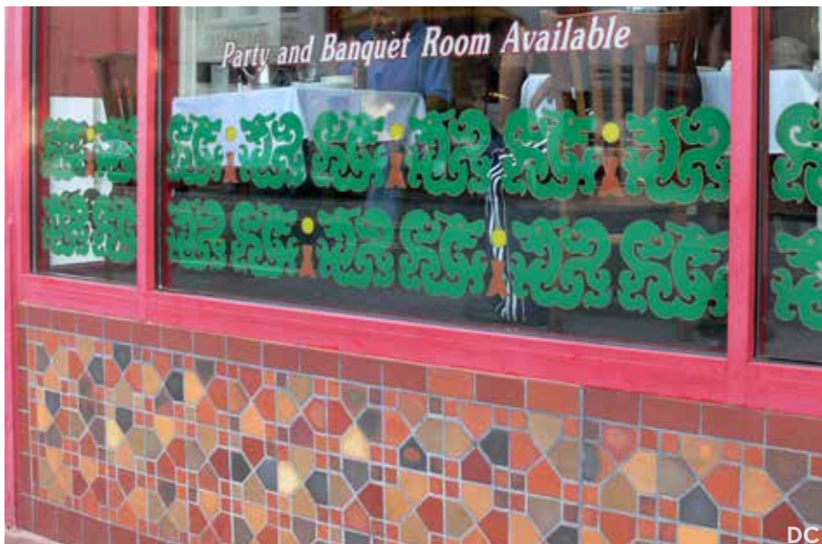
Ceramic tile on the exterior of commercial buildings provide intense color and can be highly reflective.
