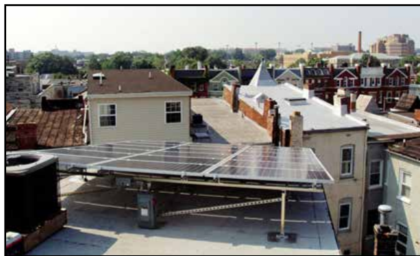
Photovoltaic installation on a District rooftop
